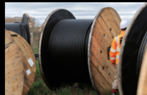
The Forterra Solar Farm Construction is underway at the site of the Forterra Solar Farm in Tils, Nottinghamshire.
